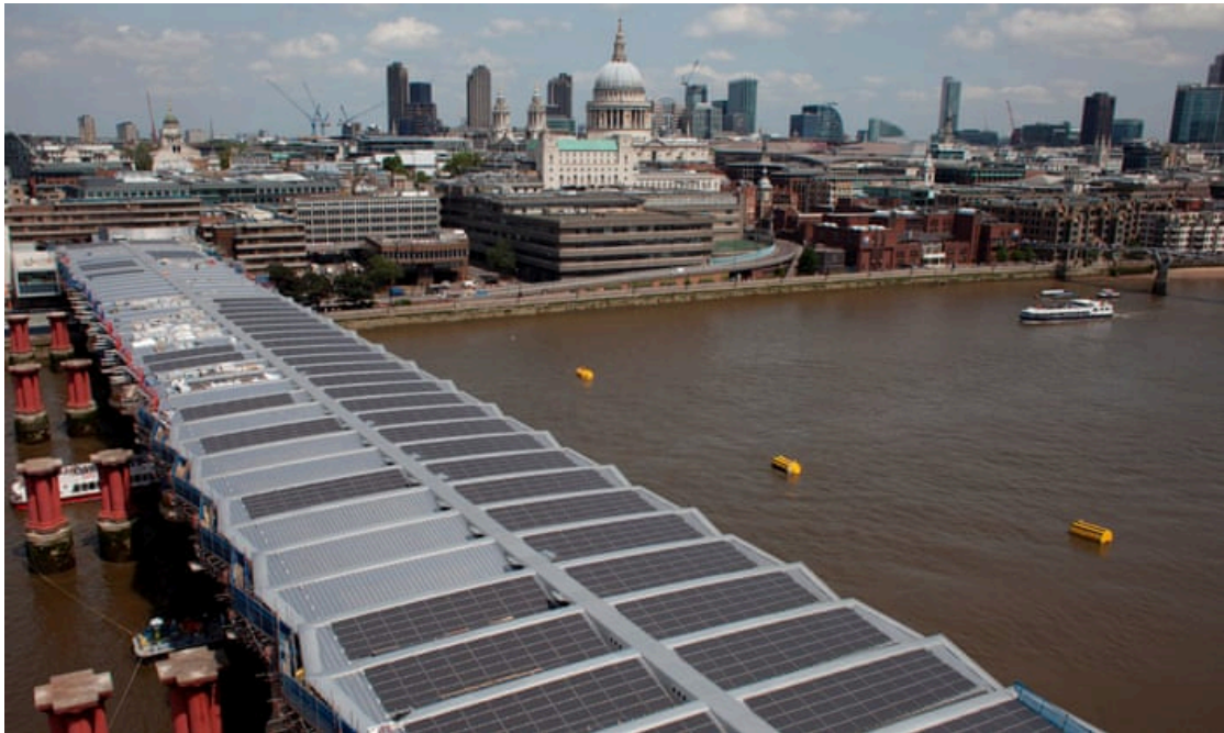
Photovoltaic Panels Blackfriars Bridge
